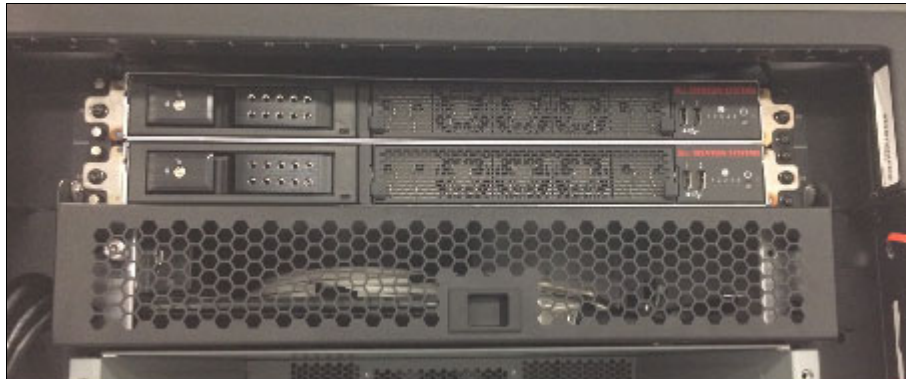
Figure 10-14 HMC and SE server location (front view)
