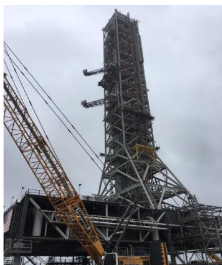
A view of the Mobile Launcher under construction at NASA's Kennedy Space Center in Florida in January 2018.
