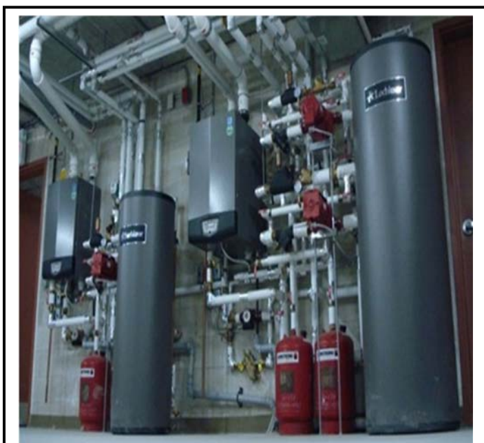
The MSFC Steam Distribution System is the second of a two phase project to convert buildings to a more efficient natural gas fired boiler system that reduces operating and maintenance costs.
