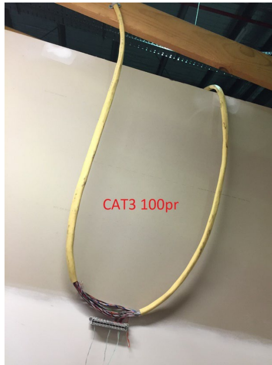
Figure 4 - CAT3 multi-pair riser cable.
