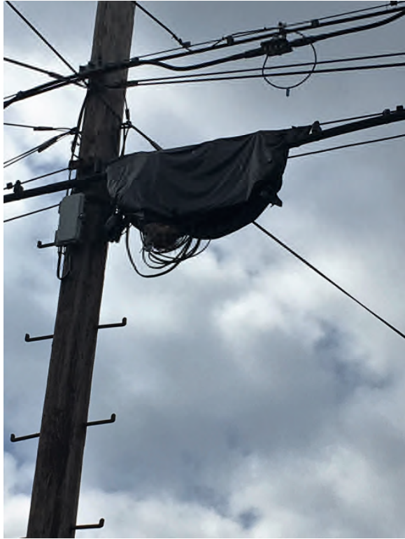
Picture 3: Improper cable repairs, wires service wires hanging out from damaged plastic wrapping over damaged cable, 643 Washington St., Northampton, Sept. 2016
