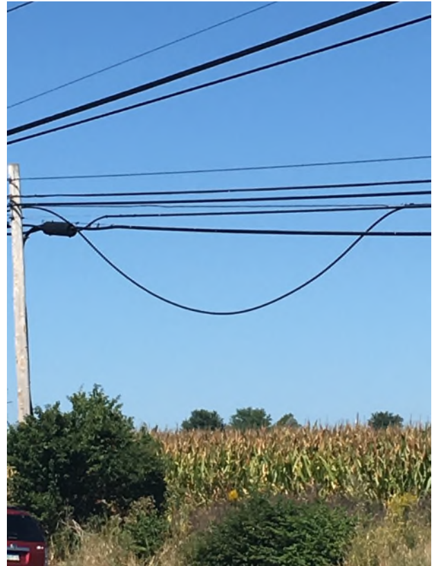
Picture 2: Line sagging below clearance, Route 342, Allen Township, Sept. 2016
