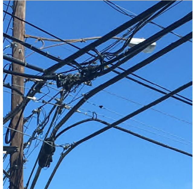
Picture 4: Failure to repair damaged cable, coupled with a failure to provide technicians with enough time to do the work properly and safely, 4th and Broad Streets, Emmaus, Sept. 2016.
