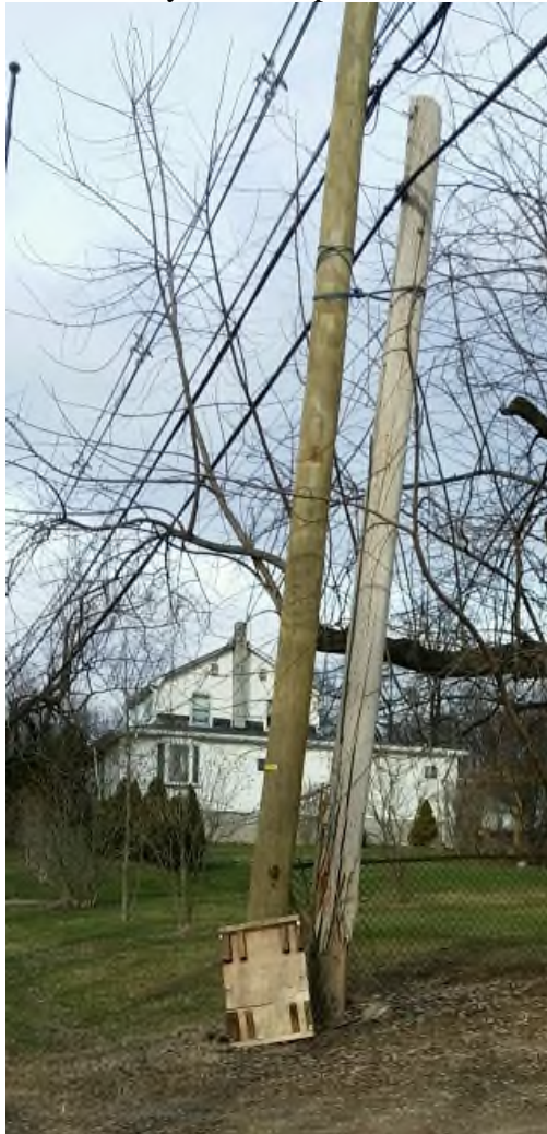
Picture 1: Broken pole, Steinruck Road, Londonderry Township, Feb. 2016
