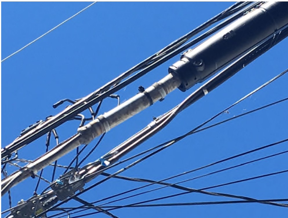
Picture 6: Lead cable exposed to the elements and improperly enclosed in a non-weather-resistant container, Milton Street, Catasaqua, Sept. 2016.
