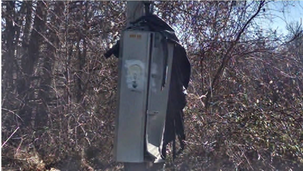
Picture 5: Damaged cabinets impair service and provide a home for nesting animals and insects, S. Birdell Rd., Honey Brook, Jan. 2016.
