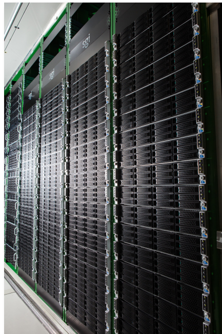
Pictured are the computational nodes inside of modular datacenter.
