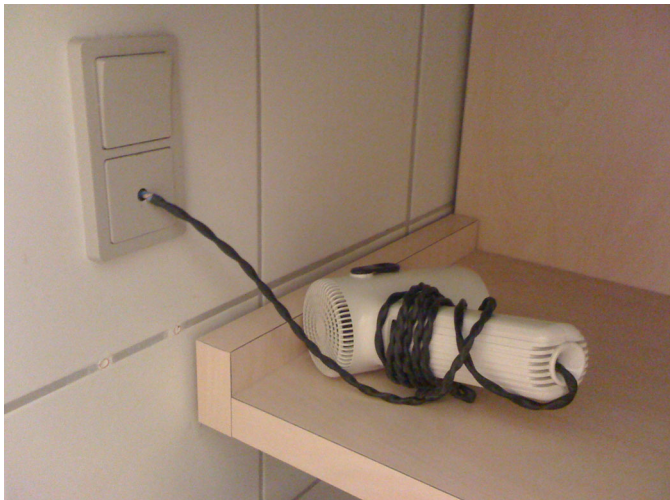
Figure 1.4 In a cheap hotel room, you might find the hair dryer wired directly into the wall outlet. This is equivalent to using the common practice of writing tightly coupled code.
