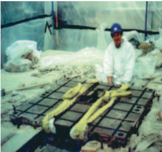
Work in progress in the containment tent erected over the core area
