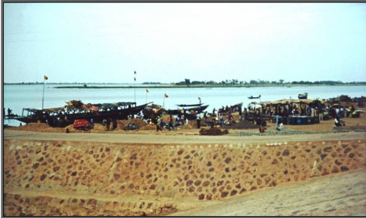
Image 8: Embankments in Mopti (financed under the Urban Development and Decentralization Project). Mopti is a major center of economic activity.
