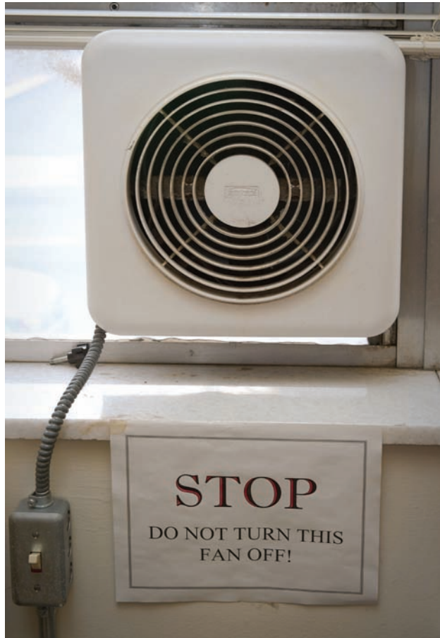
Figure 7.1 Exhaust Fan Used for Distributing Air
