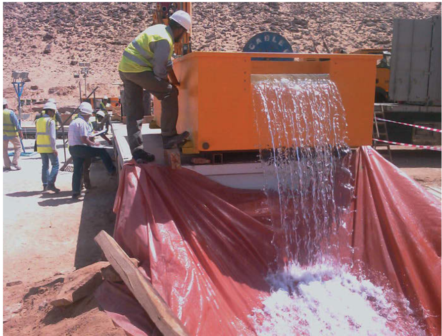
Photo 3. Pump testing in the new well field in the Rum-Saq aquifer of southern Jordan. (Photo credit: A. Andruszkiewicz)
