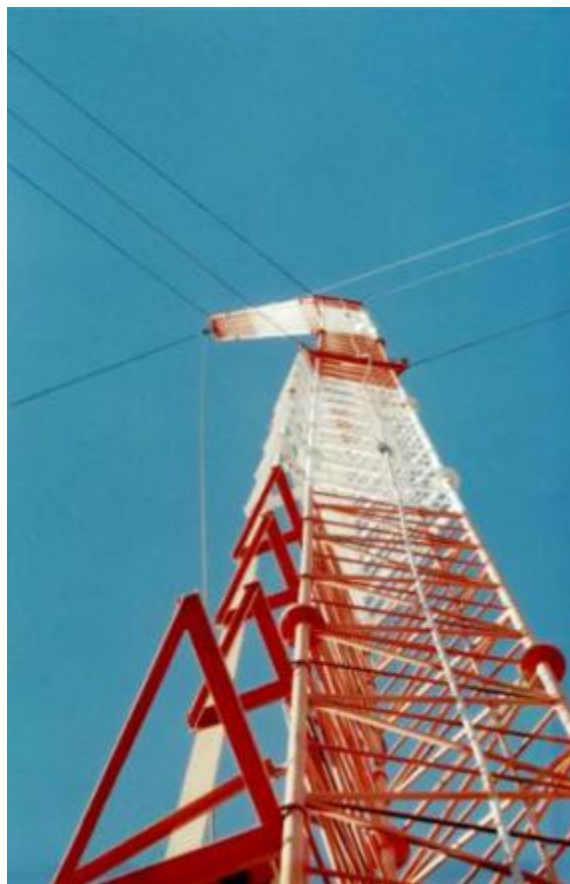
Fig. 21. A view from the ground of Tower 7 after the 2001 insulator pin failure.
