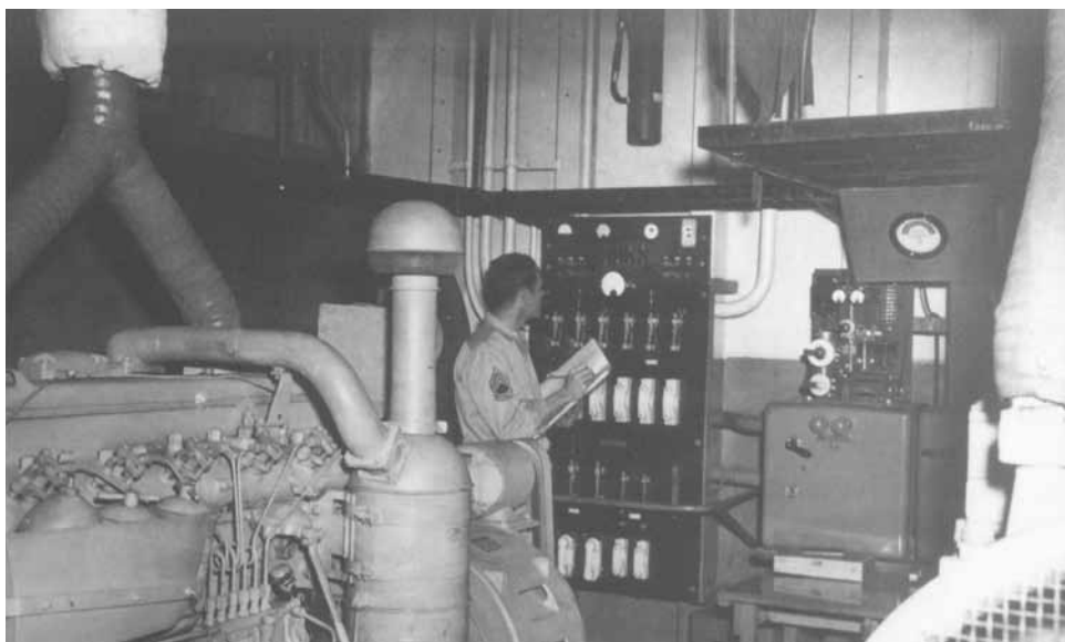
GI checks dials in the power room aboard the Apache.
