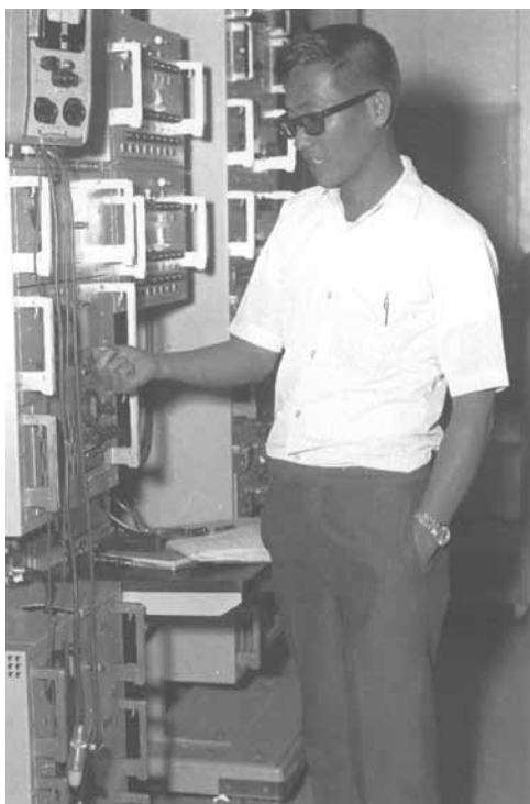
Technician from Page Communications Engineers checks equipment at the Long Binh IWCS site.
