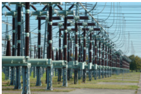
Power Utility Automation
